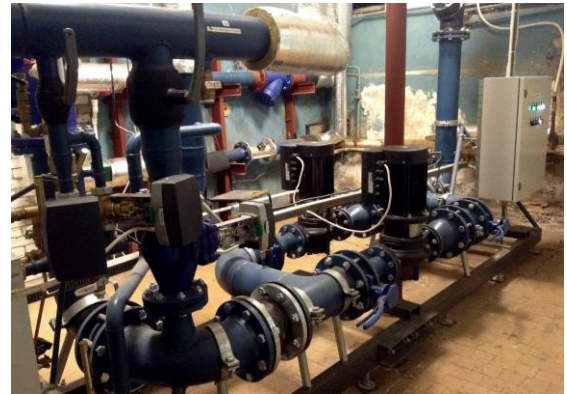
Fig. 7. Individual thermal unit in the Hidrokorpus-2.
