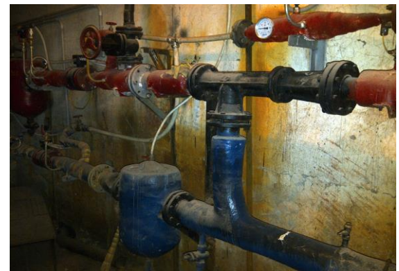
Fig. 8. Previous individual thermal unit in the Hidrokorpus-2.
