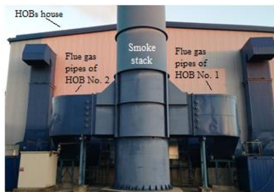
Fig. 7. Connection of HOBs No. 1 & 2 flue pipes to the smoke stack at CHP-1.
