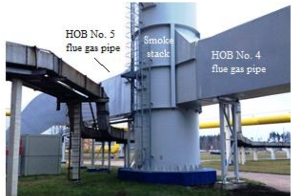
Fig. 9. Connection of HOBs No. 4 & 5 flue pipes to the smoke stack at CHP-2.
